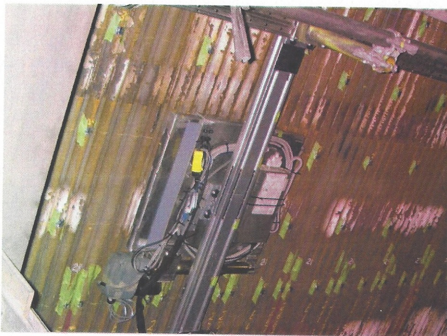
The Digital Detector Array, which captures the X-ray image, must stay precisely opposite the X-ray machine on the other side of the boiler wall.
